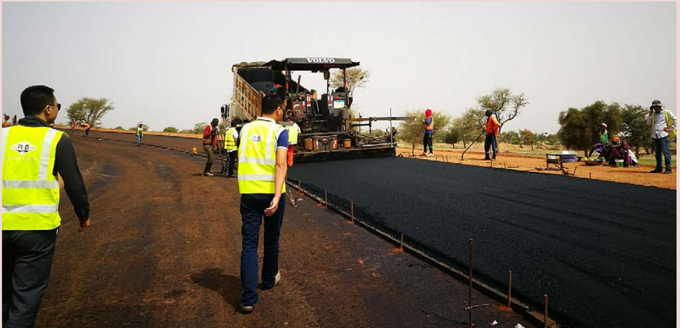
Construction of the ILA Tours highway by China Road and Bridge Corporation (CRBC) in Thiès, Senegal. Credit: Yifan Yang.
